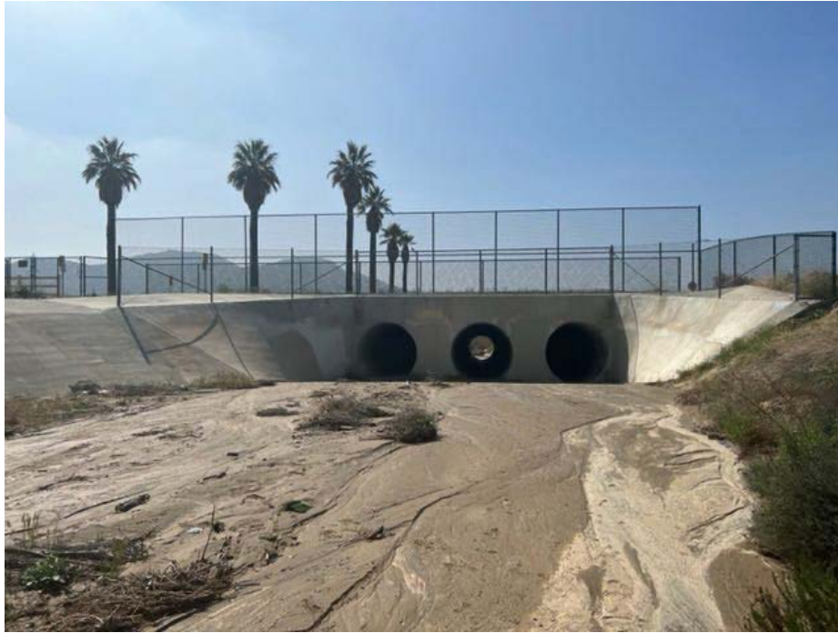
Photograph 1: South-facing view of Reach 1, from Photo Point 1, where three concrete-encased culverts pass under Cottonwood Avenue.
