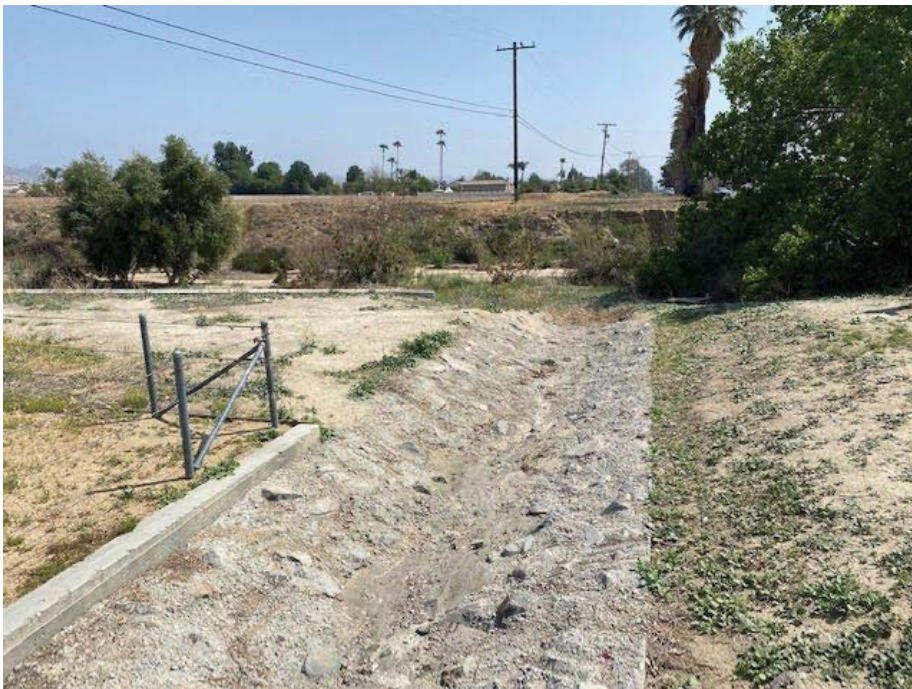
Photograph 30: East-facing view of concrete swale that runs east-west at the south end of the intersection of Bay Street and Quincy Street, ultimately emptying into Reach 5 of the channel.
